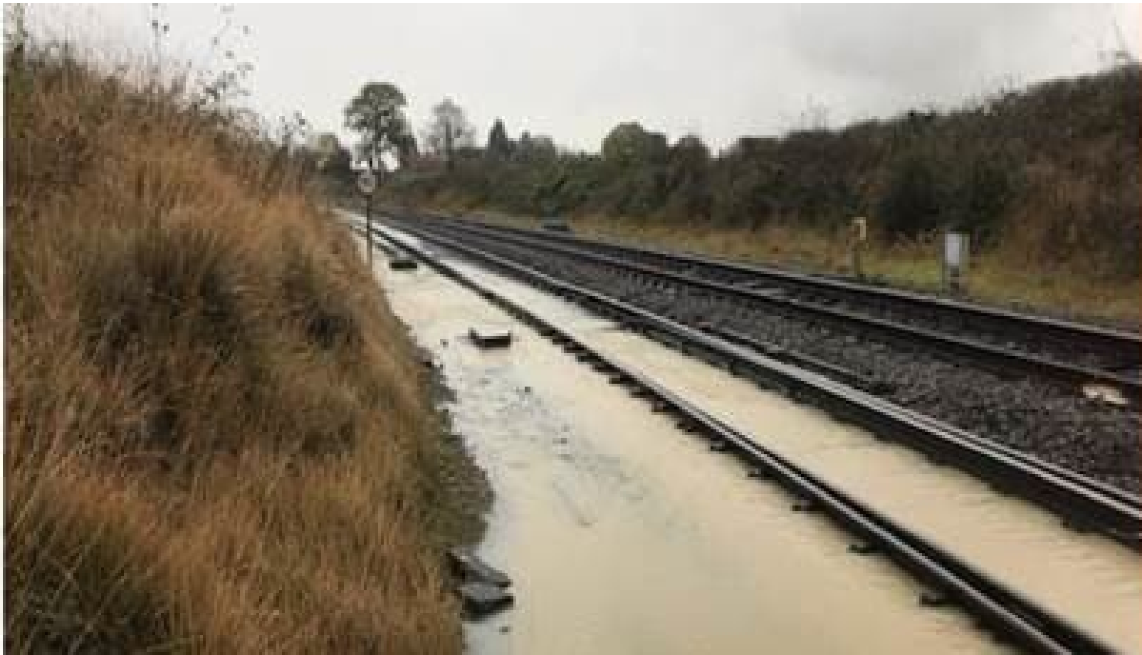
Flooding on the tracks at Bromsgrove
